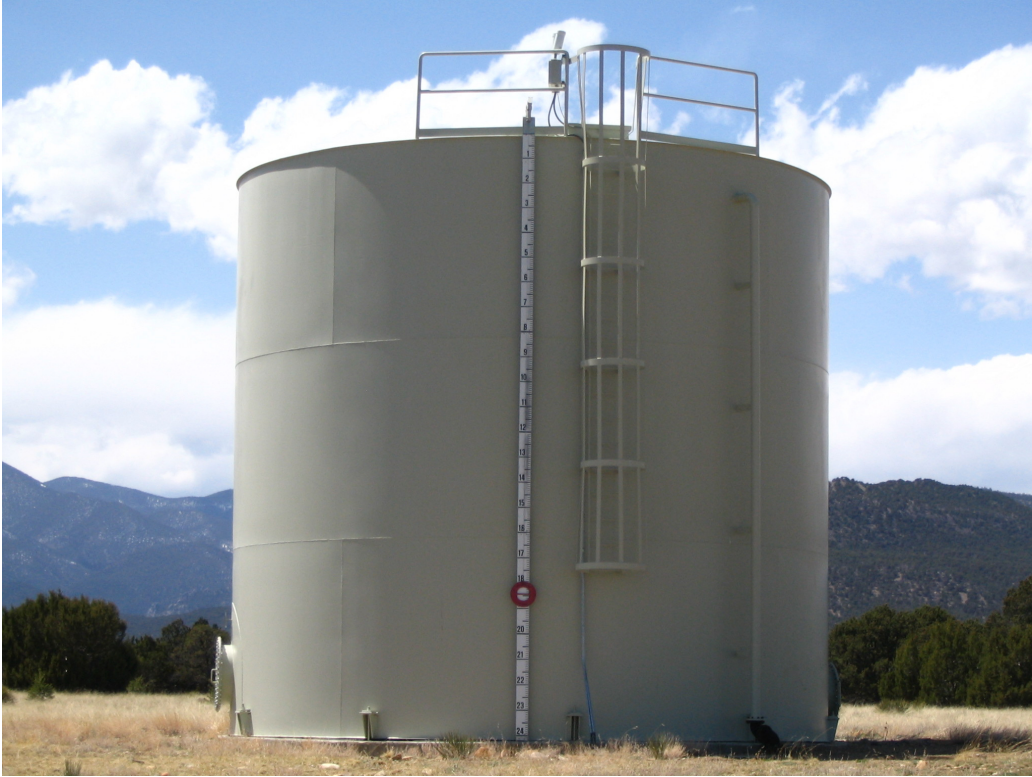
Figure 5 - Raw Water Tank
