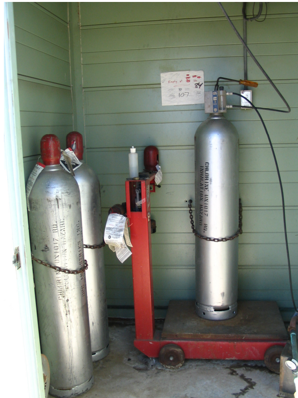
Figure 10 – Chlorine Gas Tank
