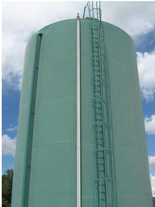
Figure 14 – Lambert Heights Potable Water Storage Tank
