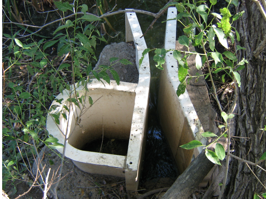
Figure 11 – Effluent Parshall Flume
