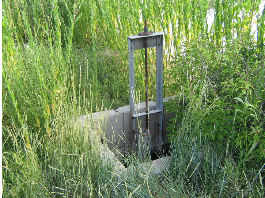
Figure 9 – Lagoon Effluent Head Gate
