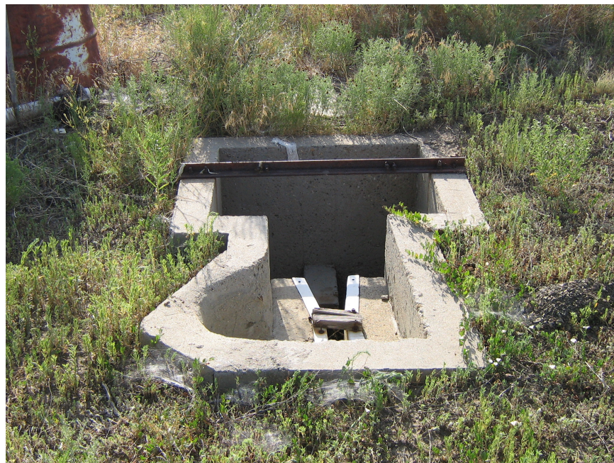
Figure 8 – Lagoon Influent Headworks
