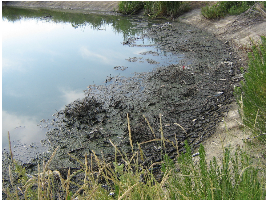
Figure 4 – Waste Deposited on Concrete Freeboard
