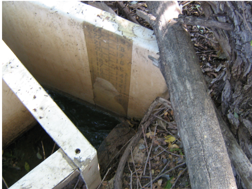
Figure 12 – Detail of Insufficient Level Reading in Effluent Parshall Flume
